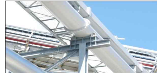
Air Slide Pipe Girder
