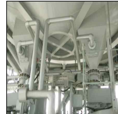
FA relay storage (Hopper·Transportation Chute)
