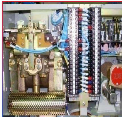
362kV GIS Pneumatic pressure TYPE
