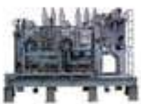
Hydraulic Power Unit (HPU)
