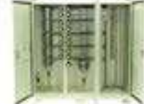
Solenoid Valve Cabinet
